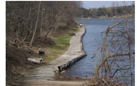
The main dock cleared of debris, tires on, bumpers to go, repairs partly done to sinking section
