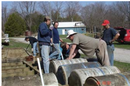
Never-ending dock repair. The floating docks for the sailing school will be replaced in the future (hopefully with the grant that has been applied for over the winter)
