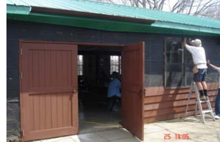
Hans Schaffner and crew replace the siding along the full east wall. Hans crafted the fine new doors. A kitchen window was replaced. All windows were trimmed as needed. A fresh coat of paint and...Bob's your uncle!
