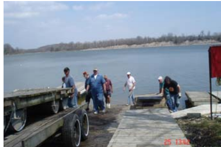
Floating the docks. It took a while to find the docks anchors and to secure them. New ramps in place!
