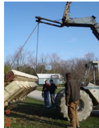
Thanks again to Dietrich Steel and brothers Steve and Alan for supplying the equip to flip the barge for repair - and move dock sections
